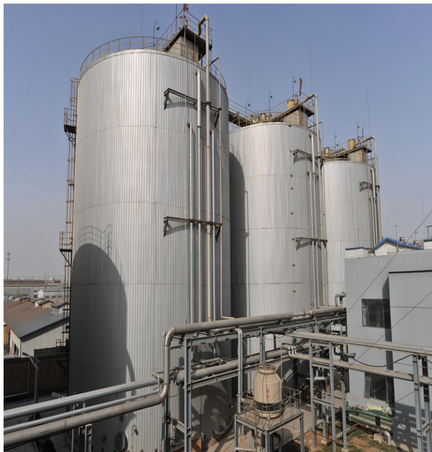
华药菌渣厌氧发酵设施 (5000m 3 *3) Chemicals' bacterial residue anaerobic fermentation devices (5000m 3 *3)
