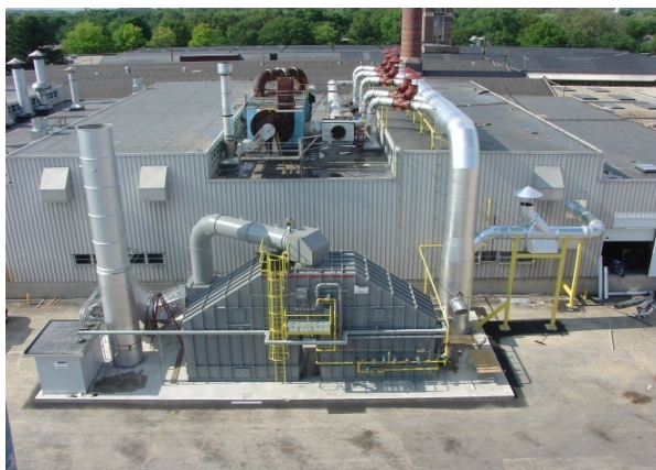
RTO蓄热焚烧
